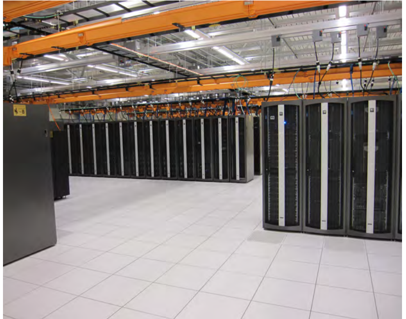
University of Wyoming ITC Data Center
